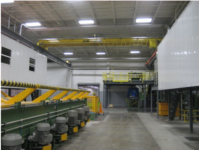
5 ton double girder crane and runway system
