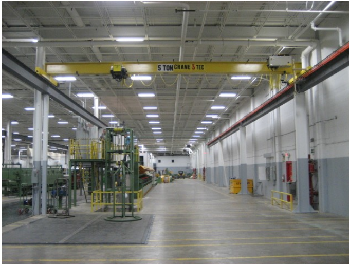
5 ton crane and runway system
