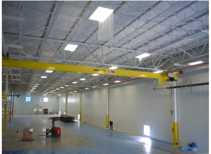
5 ton under hung crane and runway system
