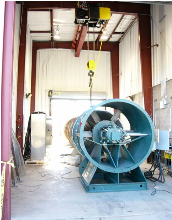
15 Ton indoor monorail system
